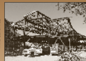
Following completion of a ring road around most Quissett Campus lab buildings at the end of 2002, construction began for a new Biogeochemistry Building, above, and a Marine Research Facility. Two additions to the McLean Laboratory and a variety of infrastructure improvements were also initiated. In Woods Hole village, a 2004 addition to the Blake Building expanded Deep Submergence Laboratory facilities.
