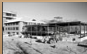
In 1989, the first addition to Clark Laboratory was occupied, and this extension to it was being framed.
