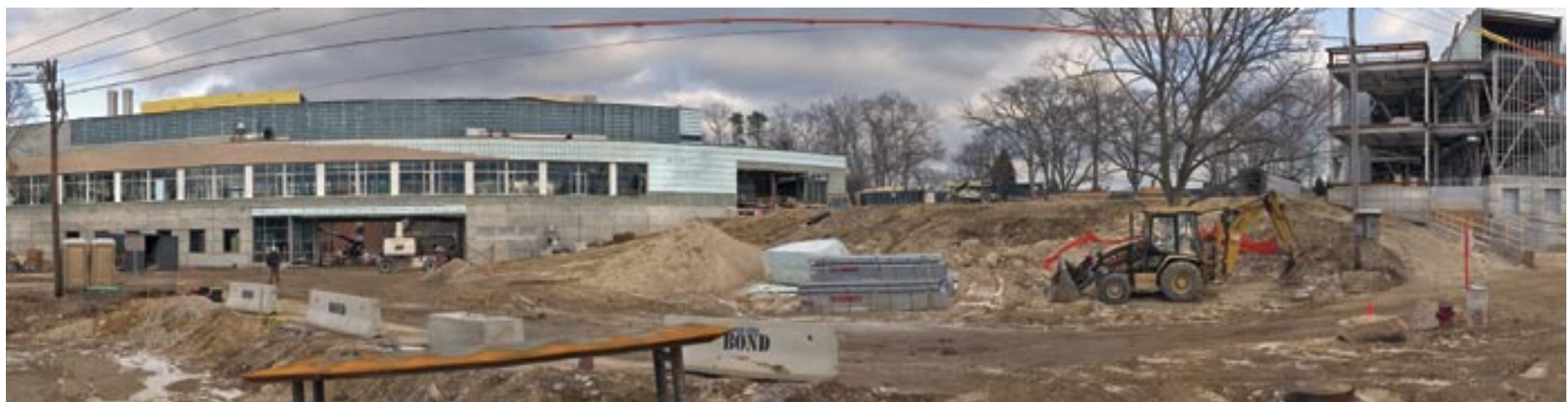
The new Marine Research Facility, left, and Biogeochemistry Building rising on the Quissett Campus in December 2004.
