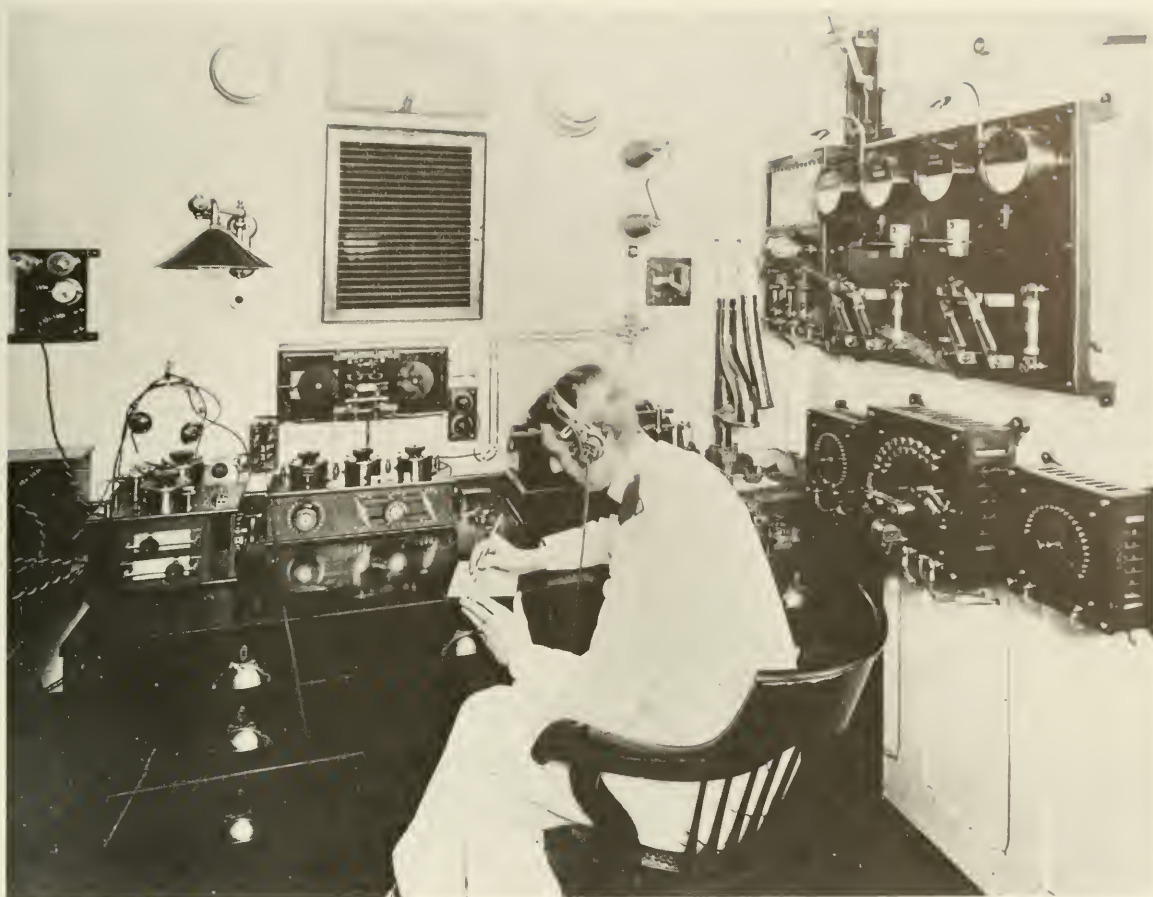
Marconi Marine 1912 installation, as fitted in the wireless room of the Titanic. At left is a valved receiver with headphones; fitted to the wall is the magnetic detector and, beneath this, the Marconi/Franklin multiple tuner; partly obscured by the head of the operator is the 10 inch induction coil spark transmitter. On wall at right are the controls of the power generator, housed in the adjoining cabin. (Photo courtesy The Marconi Company, Ltd.)
