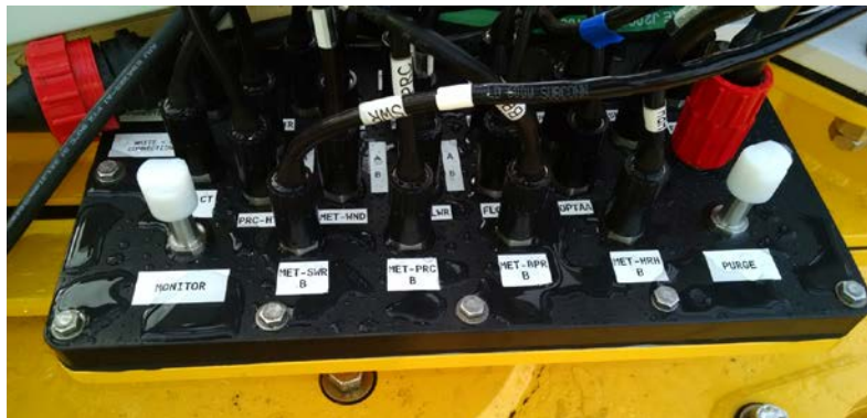
Figure 7: Monitor and Purge Ports
