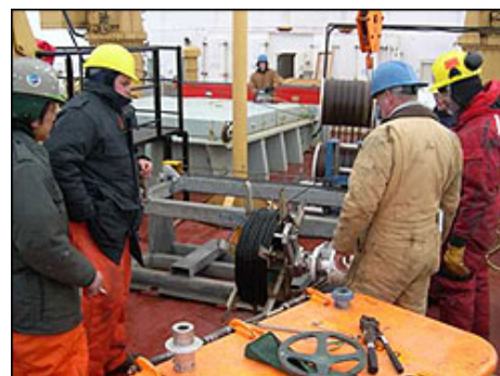
Using a specially designed dual capstan winch to reel in over 3000 m of mooring wire rope cable.
