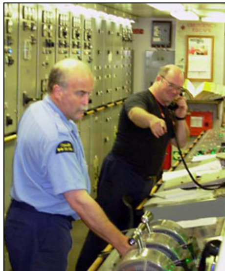
The control room is the heart of the Louis . Here Engine Room Technician Dave Ramsey and First Engineer Michael Willis monitor the Louis ' powerful propulsion system.
