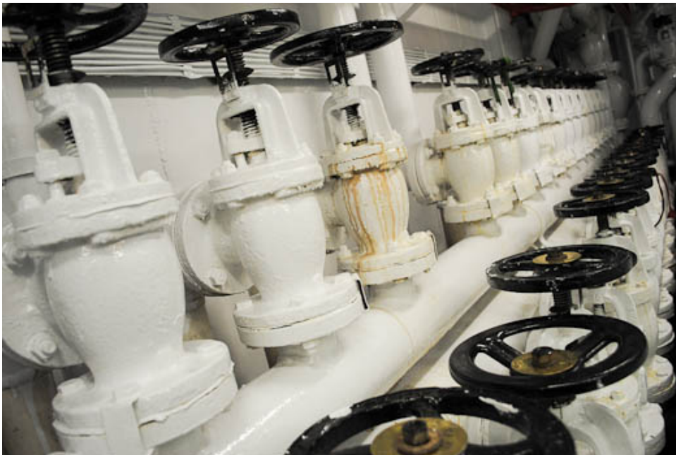
Each of these valves distributes fuel to a different tank.
