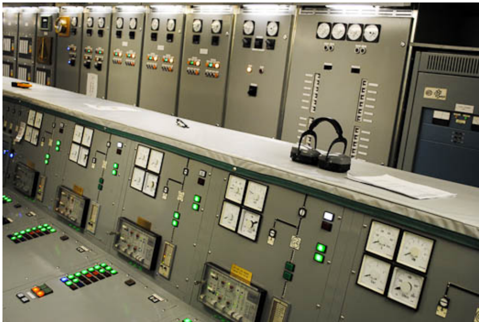
Where it all goes down. In the control room, engineers monitor thousands of separate components of the ship's electrical system.
