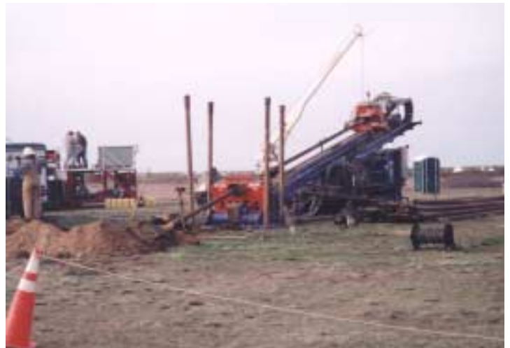
Fig. 2 Two horizontal crossings (626m and 205m) were drilled from one entrance pit.
