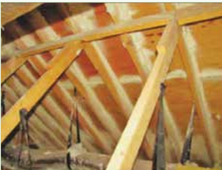
Figure 4-5. Spray polyurethane foam is used to add strength between the rafters and the plywood sheathing. This method can be used to strengthen existing roofs and may negate the need to replace older roofs. It can also be used where fasteners are missing or at the corners of hip style roofs or the ends of gable end roofs, which are especially susceptible to wind forces. See FEMA publication numbers P-499 and P-804. Image courtesy of FEMA.
