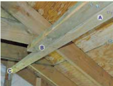
Figure 4-3. In this application of lateral bracing, the 2"x4"s are 18 inches from the ridge and connect to horizontal members that attach the opposing trusses. Not all roofs will have the horizontal members. The 2"x4"s are connected with two #14 3-inch screws (A) and overlap over two trusses (A and B). The end is connected to the gable end with an angle or L bracket (C). Image courtesy of Dennis Hwang.
