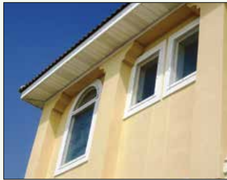
Figure 4-14. Flat impact polycarbonate panels are installed directly over windows of a coastal home. This window covering provides excellent storm protection with minimal aesthetic impact. Image courtesy of Roll-a-way.
