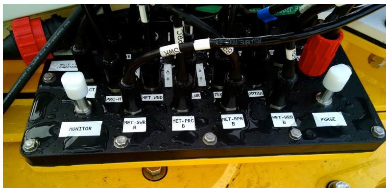
Figure 7: Monitor and Purge Ports
